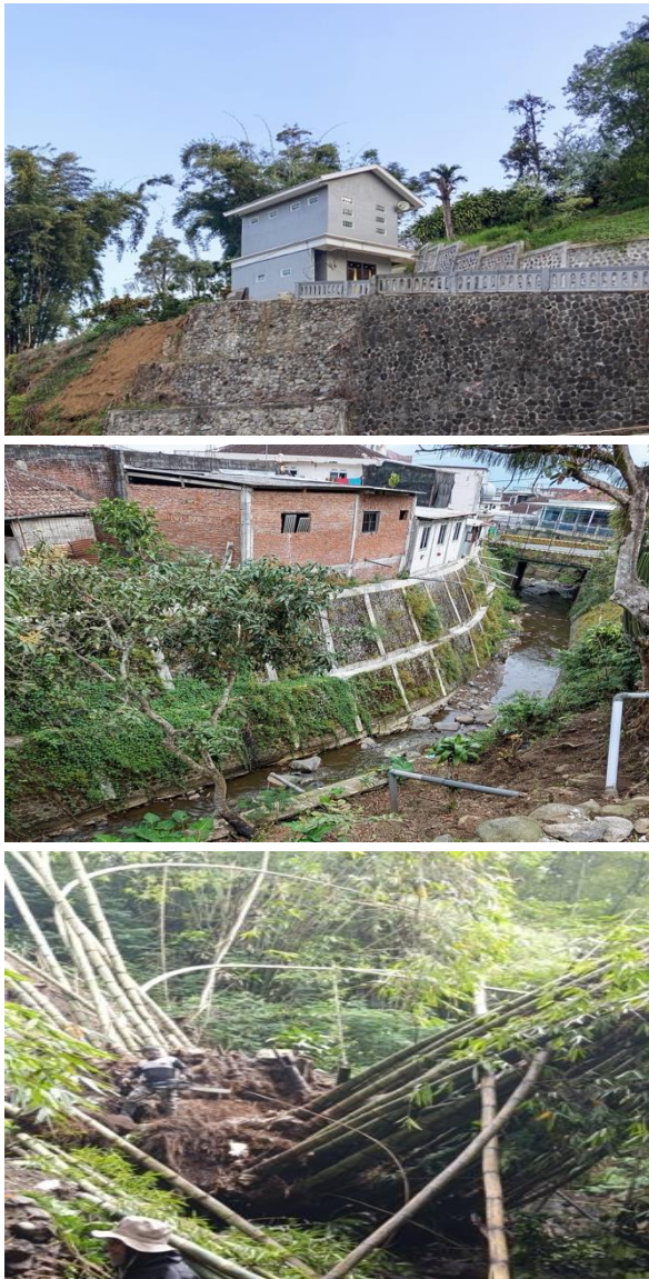
Figure 2. Documentation of the landslide event in Gempol Hamlet, Punten Village, in February 2025 (source: personal documentation)
